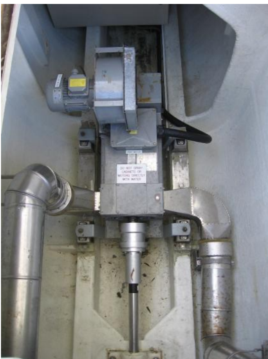
40 kW electric motor
