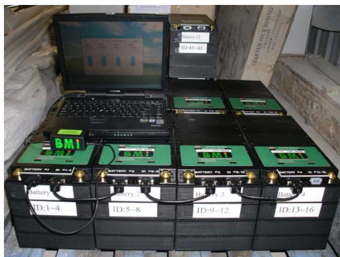
Lithium battery bank
