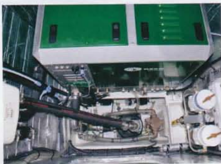
Current Sunshine – ex Bullfrog – on her first test cruise with the Torqeedo outboard motor. (top) Ossa Powerlite generator and Centrek exhaust separation system in the Fusion Hybrid. (above left)
